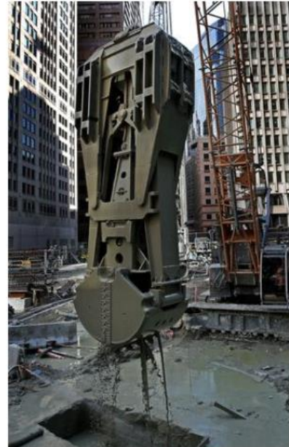
When finished, the Winthrop Square tower will be 691 feet, downtown Boston’s tallest building and the city’s fourth-tallest. DAVID L. RYAN/GLOBE STAFF/GLOBE STAFF
